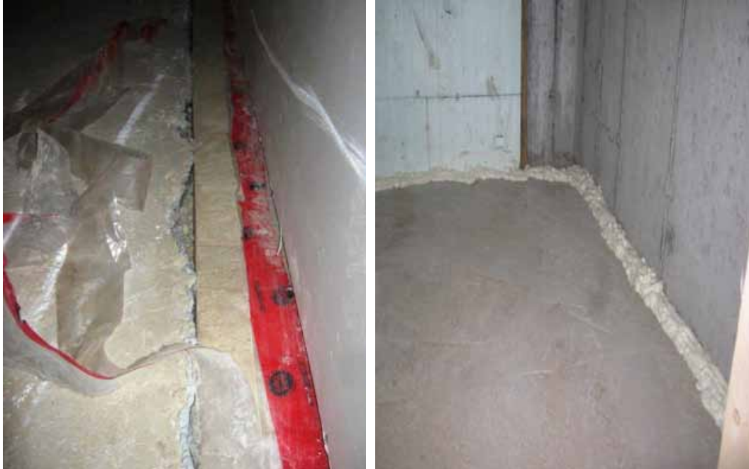
Figure 9. Example of Inadequate Sealing of Slab Edges Figure 10. Example of Slab Edges Sealed with Spray Foam
