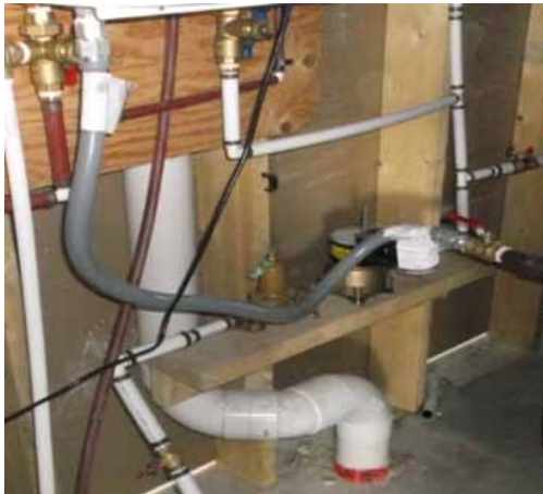
Figure 1. Example of Pipe Not Labeled
