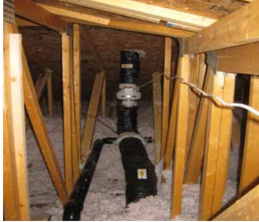
Figure 6. Example of Pipe Venting Out Roof
