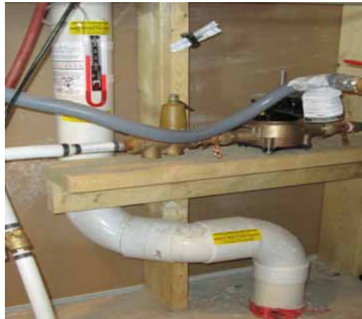
Figure 2. Example of Pipe Labeled
