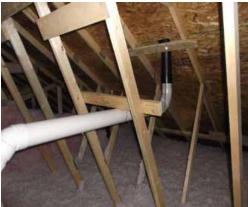
Figure 3. Example of Uninsulated Pipe
